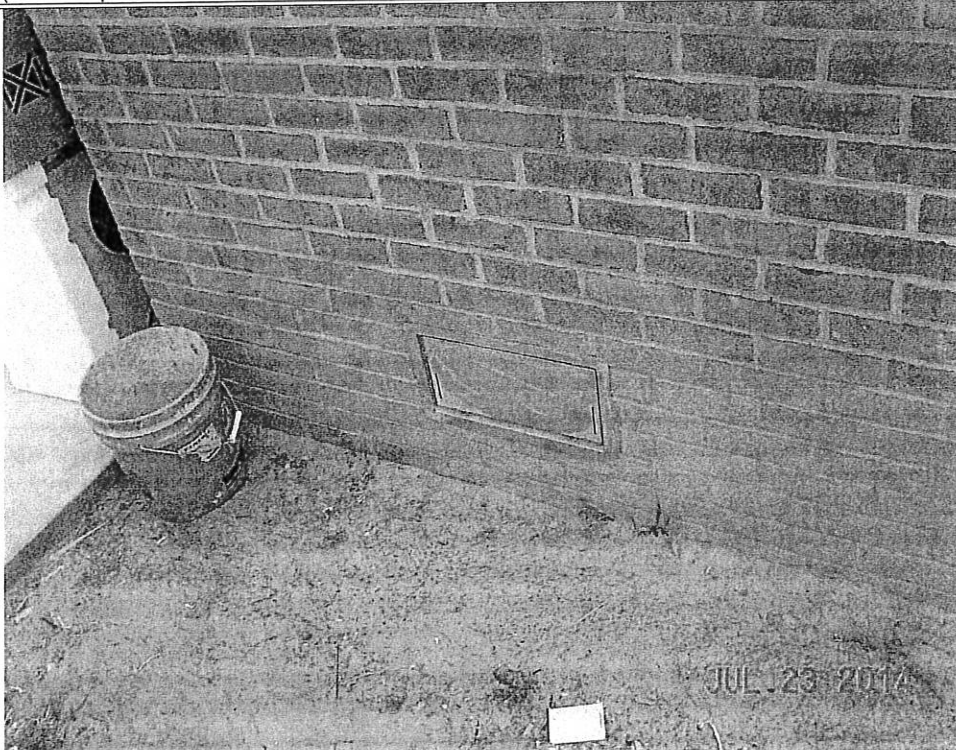
View: Engineered Flood Vent in Garage HDG #21762.01 Book 1120 / Page 54
